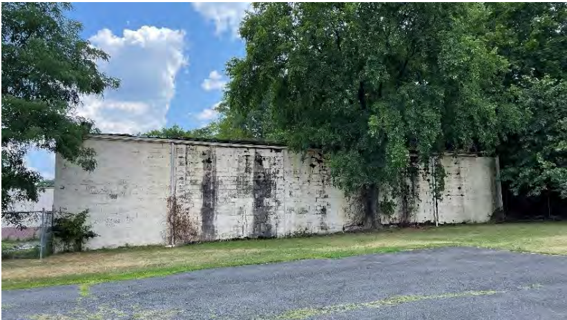
Dilapidated structure and roof from side yard.
