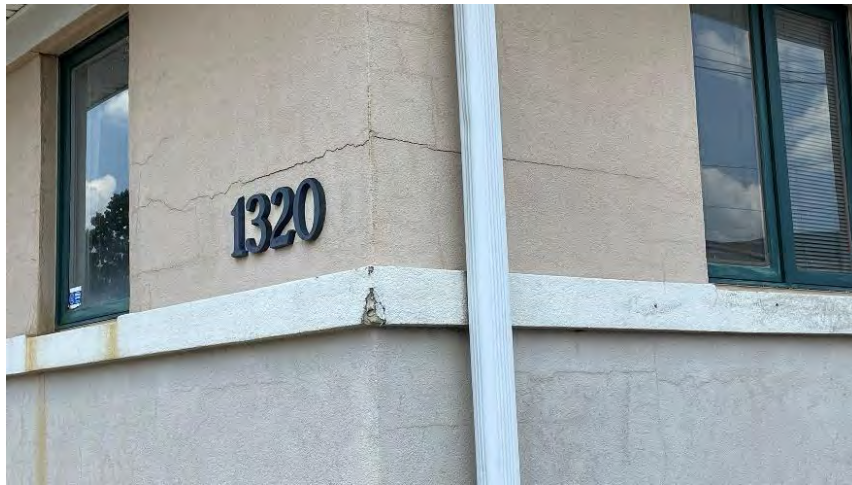
Cracks in exterior wall
