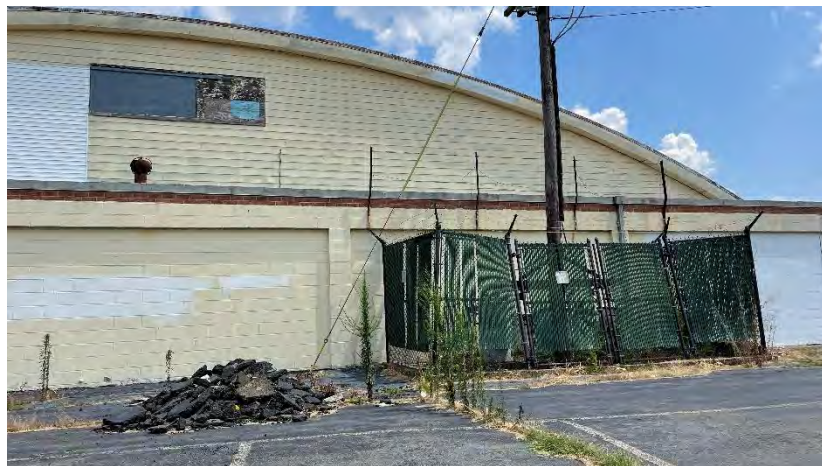
Haphazard loose building debris in rear
