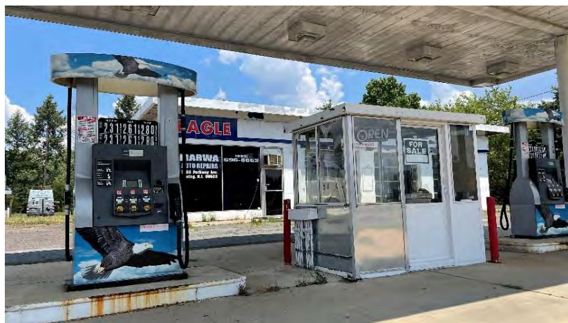
Gas pumps and service booth.
