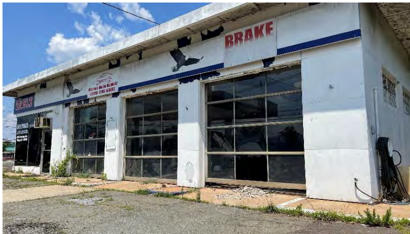
Dilapidated garage bays
