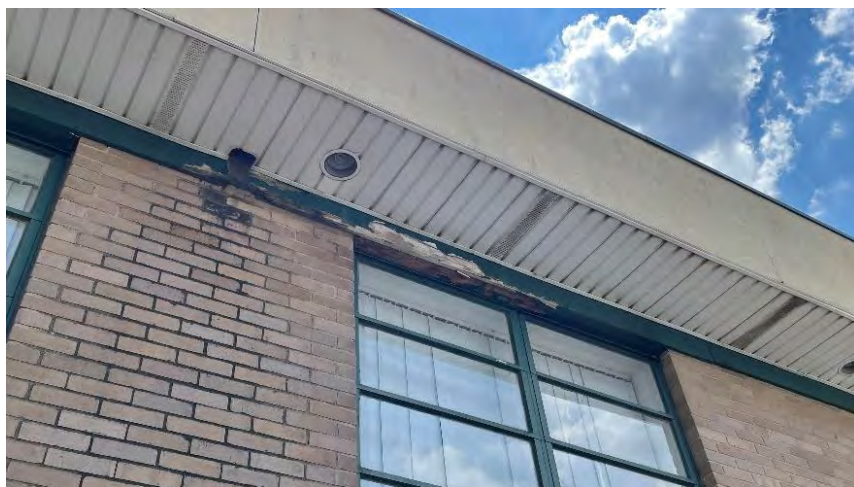
Exposed wood soffit/facia and disconnected downspout.
