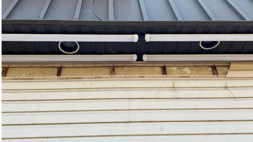
Broken vinyl siding and exposed wood framing.
